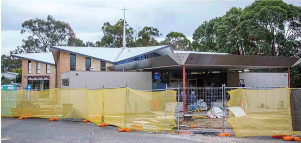
A view of the renovation project at Our Lady of the Rosary Parish, Kellyville, in August 2022. Image: Diocese of Parramatta.
